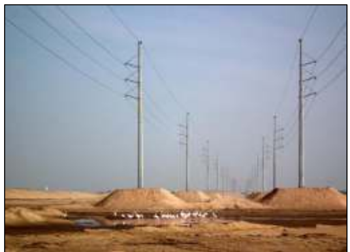
Water seepage has unfortunately attracted many birds to the areas beneath the power lines, increasing the chances of collisions when the birds are startled (photo Ann Scott)
