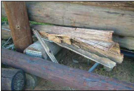
Damage caused by termites to creosoted Erongo RED power line poles at Omaruru (photo Ann Scott)
