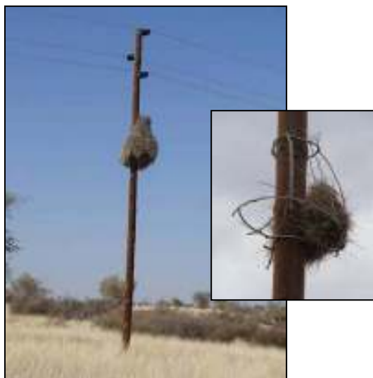
Basket (made out of old conductor wire) on Kalkpan HLPCD (horizontal line post compact delta) reticulation line, Farm Dai Gratia ( photo AC van Zyl )
