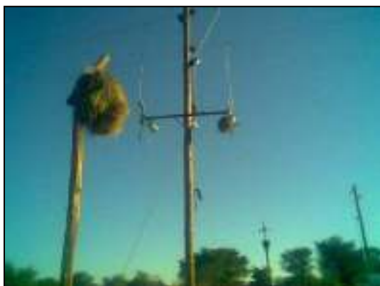
Dummy pole on Farm Eldorado (pump) on Kalkpan reticulation line, 153km from Aranos (see dummy on left, and smaller nest on the cross-arm structure; photo AC van Zyl )
