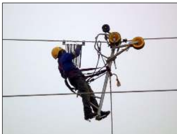
The new 132 kV Kuiseb-Walvis Bay power line has been marked as a mitigation for bird collisions (above); fitting of markers for mitigation (below; photos Ann Scott ).
