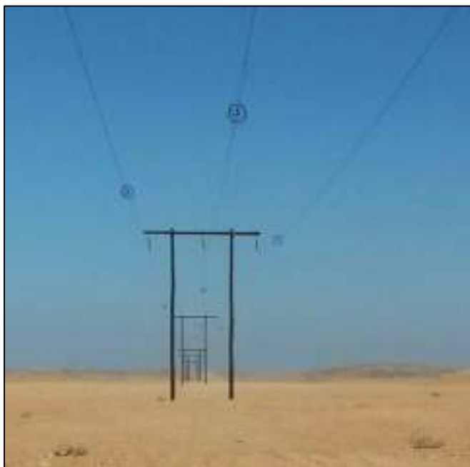
Marking of the 66kV Line re-route near Lüderitz (photos Pankratius Kondjamba, Namdeb).
